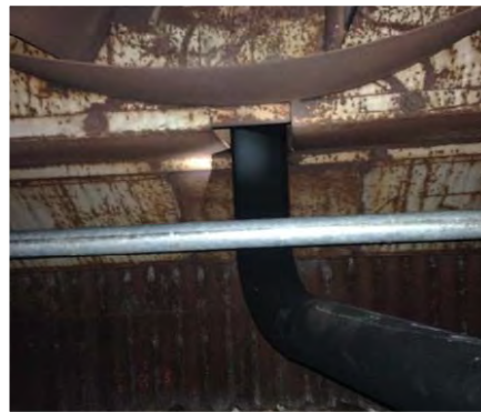
Black pipe in windbox
